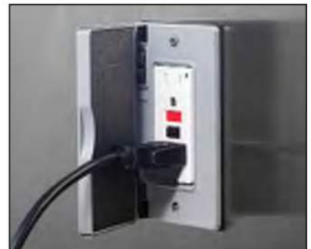
Electrical duplex receptacle with splash cover
